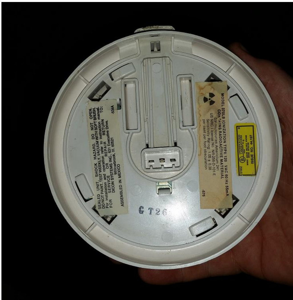
Figure 2. Smoke alarm at a small hotel in Georgia. The date code indicates the unit was at least 9 years out of date (made before 1999), the battery was removed and the power disconnected. The alarm was completely inoperable.
