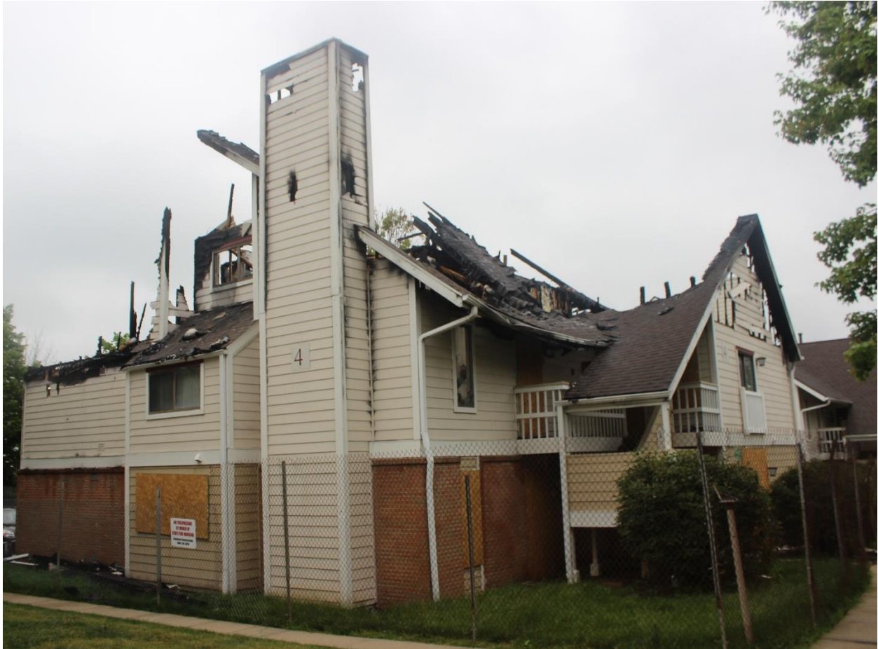
Figure 1. Recent hotel fire. One fatality, one serious injury. Lightweight construction, limited egress and faulty alarms lead to rapid fire spread and little warning to occupants.
